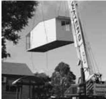
Demountable classrooms being moved to their new location on the CCAS campus.
