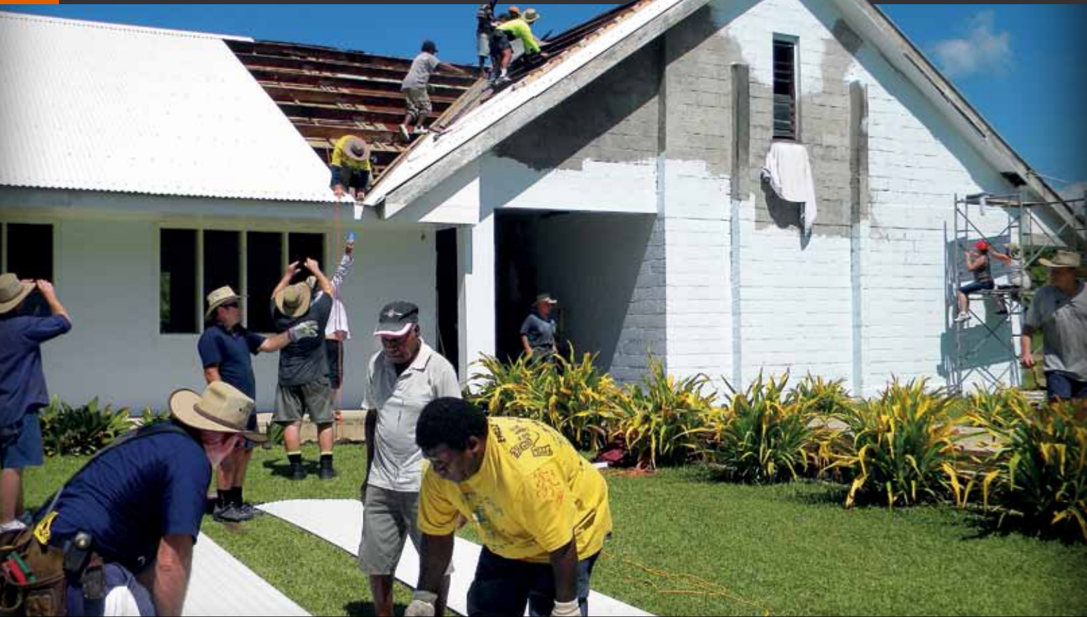
A Fly'n'Build mission to Vanuatu saw volunteers re-roof and paint the Sarakatu Church in Luganville, and complete a number of other projects.
