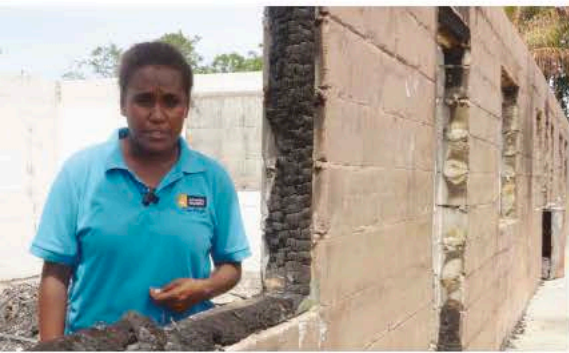
Tenakoga teacher Chareen Simbe in one of the burnt-out buildings.
