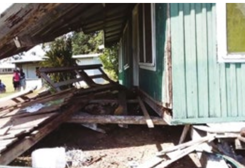
The principal’s house is off its stilts and has sustained major damage.
