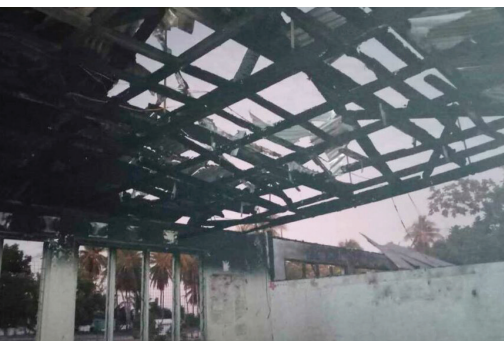
A number of administration offices and classrooms were destroyed.
