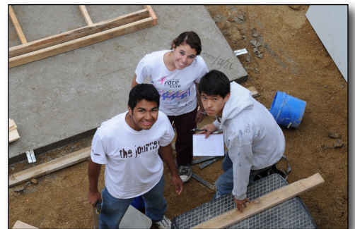
Students from EAA that have just finished pouring the slab for the foundation of a much-needed house for a family in Baja, Mexico. The framing is in process. The house was completed in four days of concentrated effort by the group of students. From left: Sammy Martinez, Kacey Hawkins and Kalani Berry.
