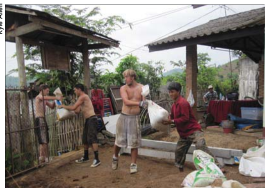
Eric Smith, Collin Monty and Alex Smith work with a villager swinging heavy bags of gravel to the top of a huge hill to mix cement for a church building project.
