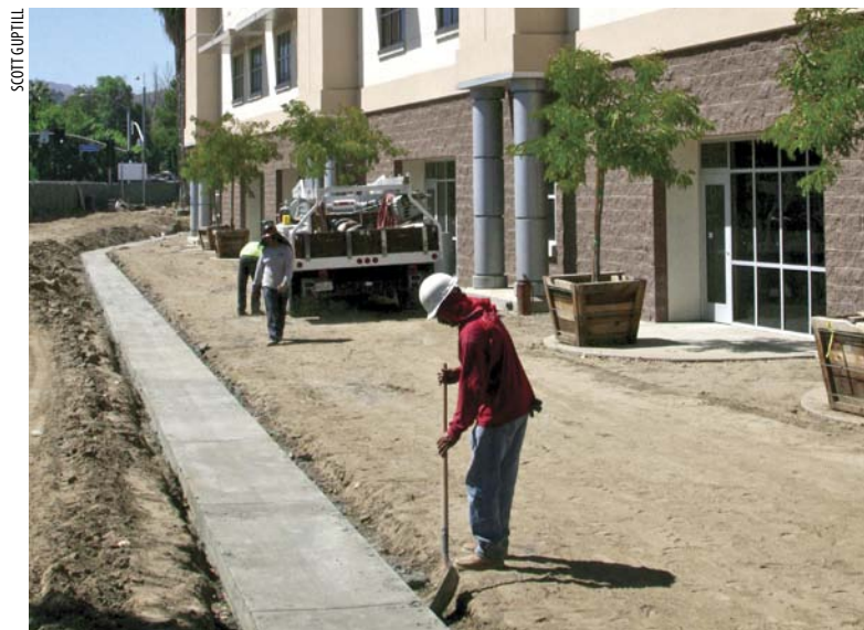
Construction workers work on the final touches by planting trees and creating the pathway along Anderson Street.
