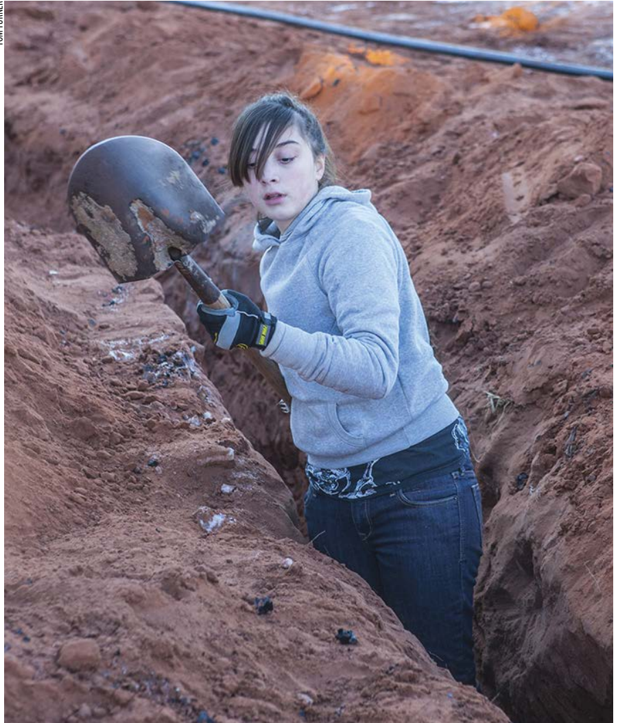
PUC students, including Miriam Petersen, spent Christmas vacation digging up frozen pipes and renovating a church in the Navajo community near Page, Ariz.
