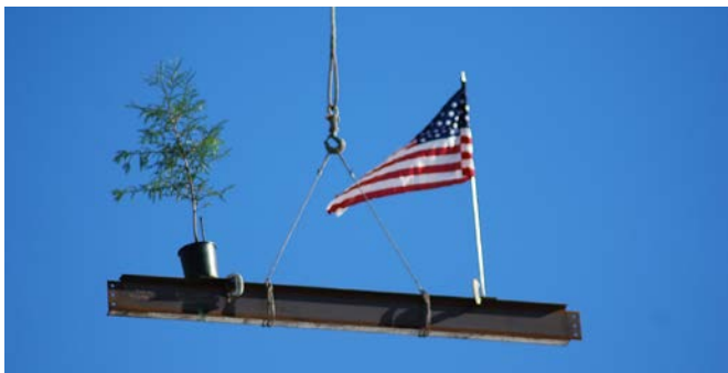
After only 13 working days on the steel frame, crews placed the final beam of the new Howard Memorial Hospital and officials held a "Topping Out" ceremony to celebrate.
