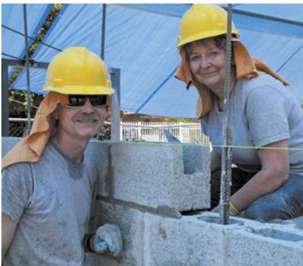
Jack and Neoma Wisdom, Paradise church members, lay block for the new school.
