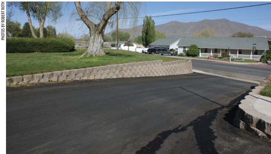
The retaining wall and paved driveway come together to create an attractive and practical new entry for the Winnemucca church.
