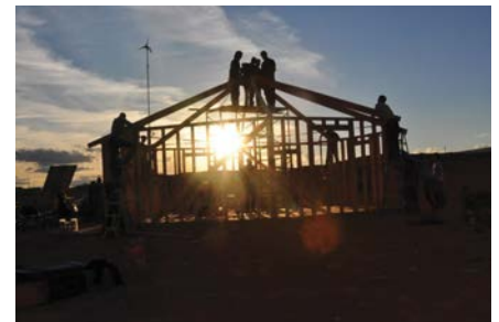
Traditional hogans were made from logs and mud. This new construction was designed by Jeremy Noble, a senior at Mesa Grande Academy.
