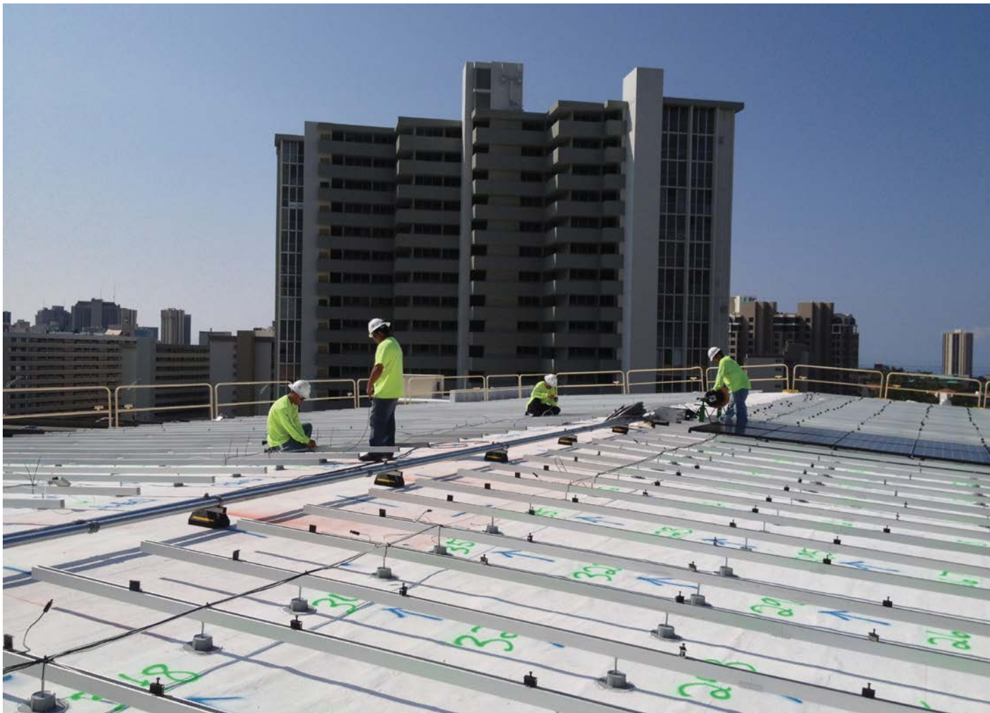
Workers install the hardware used to mount hundreds of panels on the gymnasium roof.
