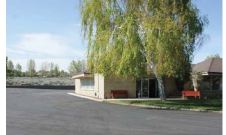
The new parking lot still needs the contractor's final touches of striping and curbing.
