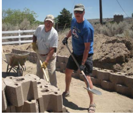
Head elder Peter Wool and Dr. David Simsek work on the retaining wall project in preparation for the asphalt.
