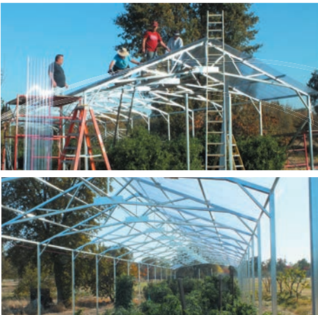
(Above) Carmichael church members build a greenhouse, using three Maranatha Volunteers International One-Day Church kits. (Photos by John Wilt)
