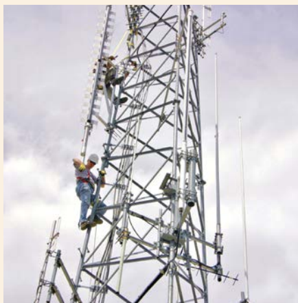
Stephen Denny (engineer, GNTV Dallas/Ft. Worth & Brazos TV) moved to Phoenix for a month to volunteer hundreds of hours to get three new Arizona TV stations on the air. Here, he and Moses Tyler secure the antenna on the tower in Flagstaff.
