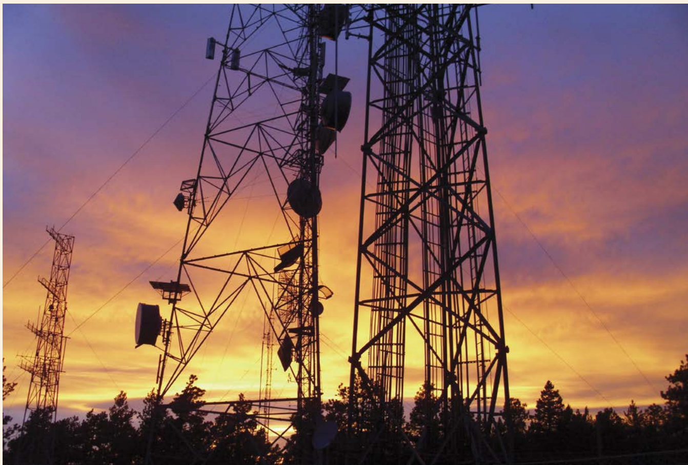
GNTV crew members were happy to complete the broadcast antenna installation just prior to sunset as Sabbath drew on.
