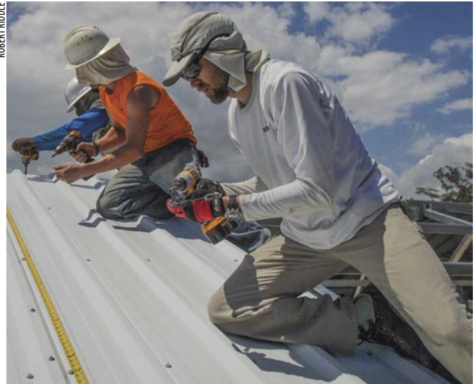
Chris Pappas, Leoni Meadows forestry supervisor (orange shirt) and Greg McCulloch, Sonora Regional Medical Center CFO, bolt roofing into trusses.
