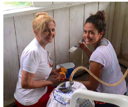
Volunteers build and paint facilities used by Adventist missionaries in Rosa de Saron.
