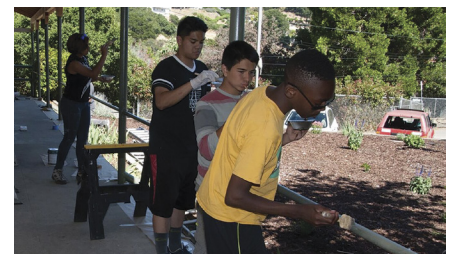
Volunteers paint the handrails and trim of an administration building at Golden Gate Academy.
