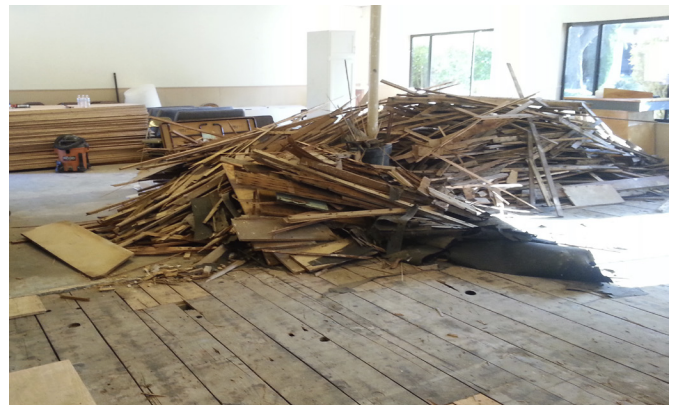
The original fellowship hall floor is demolished in preparations for its remodel.
