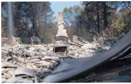
Paradise Adventist Academy loses its K-4 school building in the Camp Fire and sustains other damage.
