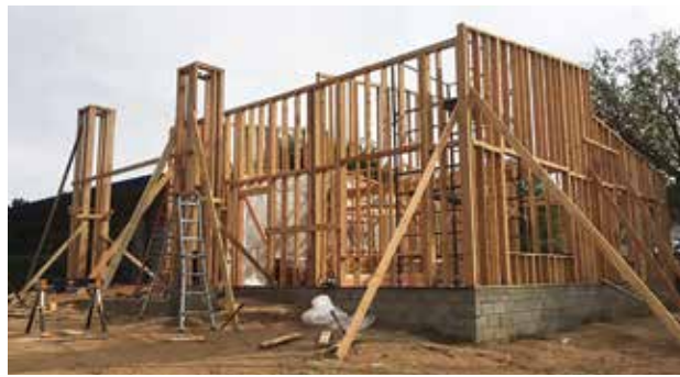
The project got underway in April 2016, nearly six months after the contract was initially signed.
