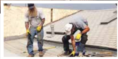
(Above) The Diamond Street Resource Center provides resources. (Inset) Pat Leo and Barry Wilkens complete major roof repairs on the building. (Right) Camelback members Barry and Terry Wilkens have volunteered their time and resources to make the DSRC a success.
