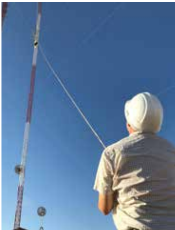
A volunteer crew member lifts supplies up to a tower crew on a hot (108 degree) Arizona desert summer day.
