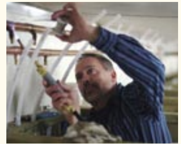
Clair Kitson, plant services director, volunteered his time to install showers in a 48-foot trailer.
