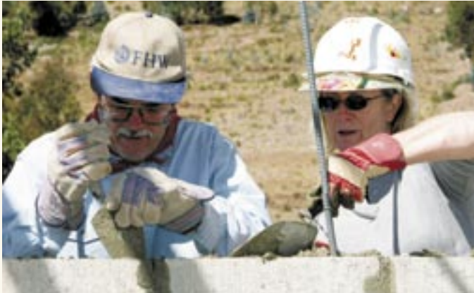
Larry Soule and Connie Rodenberg work at a new church building site in Jaillibuaya, Peru.
