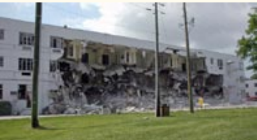
The imaging and therapy building, which housed the residence hall, in the beginning stages of demolition.
