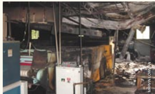
Fire began in the ironing-folding area of the Madison Academy Linen Service when lightning struck the electrical service.
