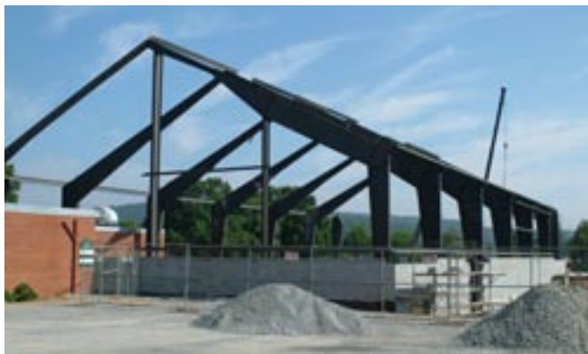
Southern launched construction of the $6.5-million wellness center in February. The new wellness center will provide a space for students to learn, live, and share a holistic healthy lifestyle. This is the University's most ambitious building project since the new science building was finished in 1997.
