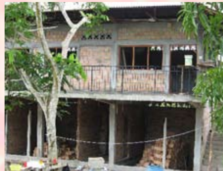
The top three rooms of the Crisis Center Dormitory are almost finished, and the bottom floor is well under way. Twelve more rooms are in the plans for this complex.
