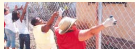
The students and staff help to install a new fence around the school.
