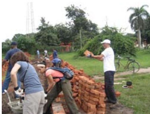
Walter Fordham (left), and Brenda, Kristen, and Keith Wood work on constructing the fence.
