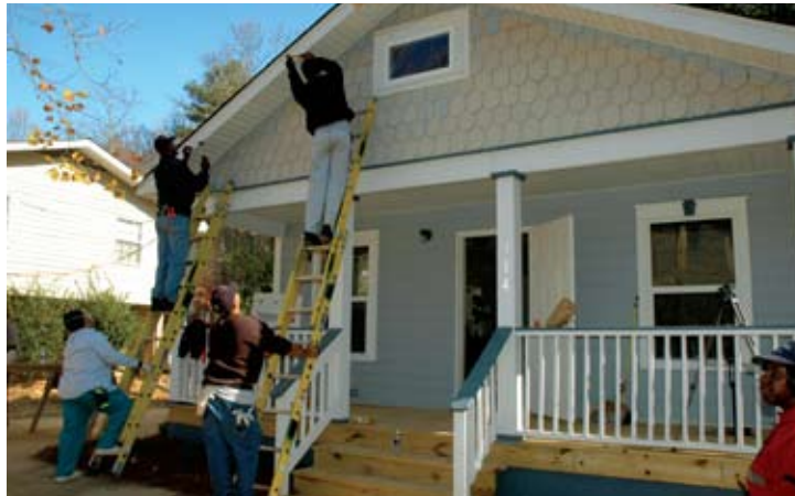
After seven Sundays of work on the Habitat for Humanity house in Atlanta, finishing touches were completed before the dedication ceremony.
