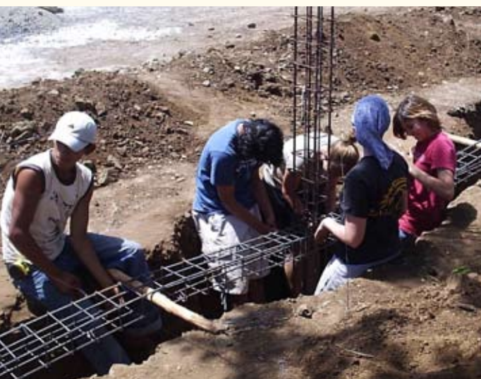
One project at the orphanage was to group rebar together by hand for the footers and columns of the maintenance building, in preparation for pouring of the cement.
