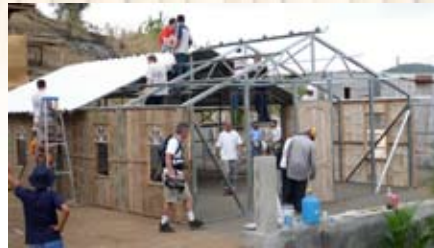
The first One-Day Church was built in Valle Hermoso, Ecuador, this July.
