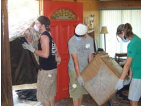
Jesse Baker, Chris Tozer, and Gabbie Clifford help empty a home of moldy furniture and belongings ruined in the floodwaters of Hurricane Ike.
