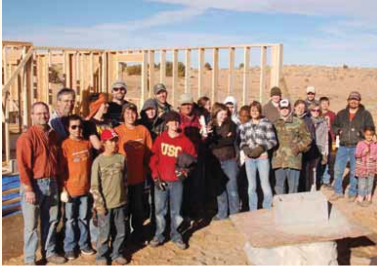
One team finished the framework for Joe Littleman's (center, wearing tan cap) house.
