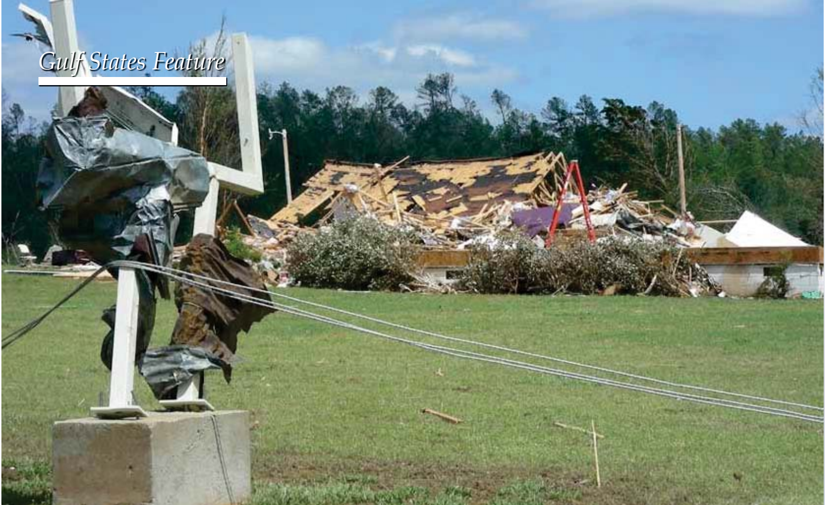
Not much was left of Piedmont Church after a tornado slammed into it on April 27, 2011.
