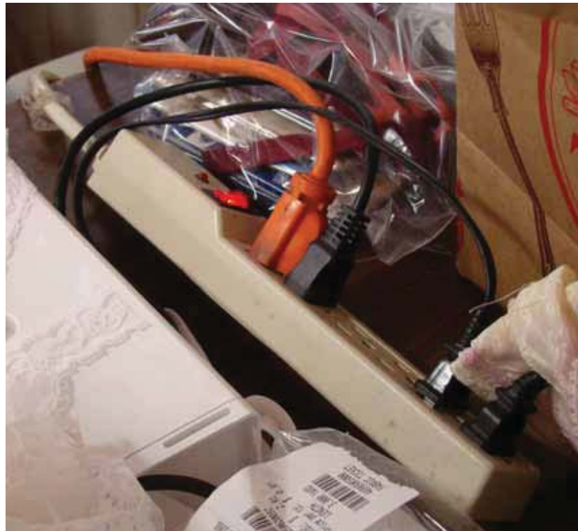
Hazardous area: This is a fire waiting to happen.
