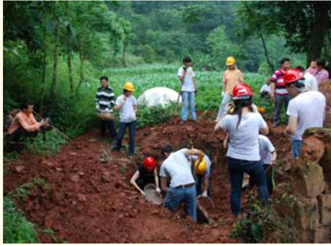
The GCA group installed seven biogas tanks. They were only supposed to install three.
