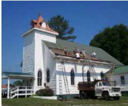
Antique metal shingles covered by layers of asphalt shingles were replaced with a new standing-seam metal roof.
