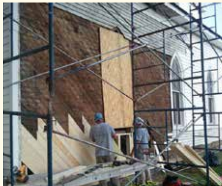
Part of the termite-damaged west wall was five inches off the foundation before being re-framed back into plumb.
