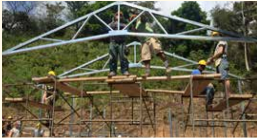
The steel structure begins to take shape with the help of students from Georgia-Cumberland Academy.
