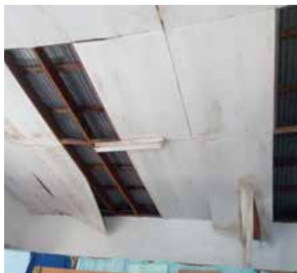
The ceiling shows signs of water damage before renovations were made.
