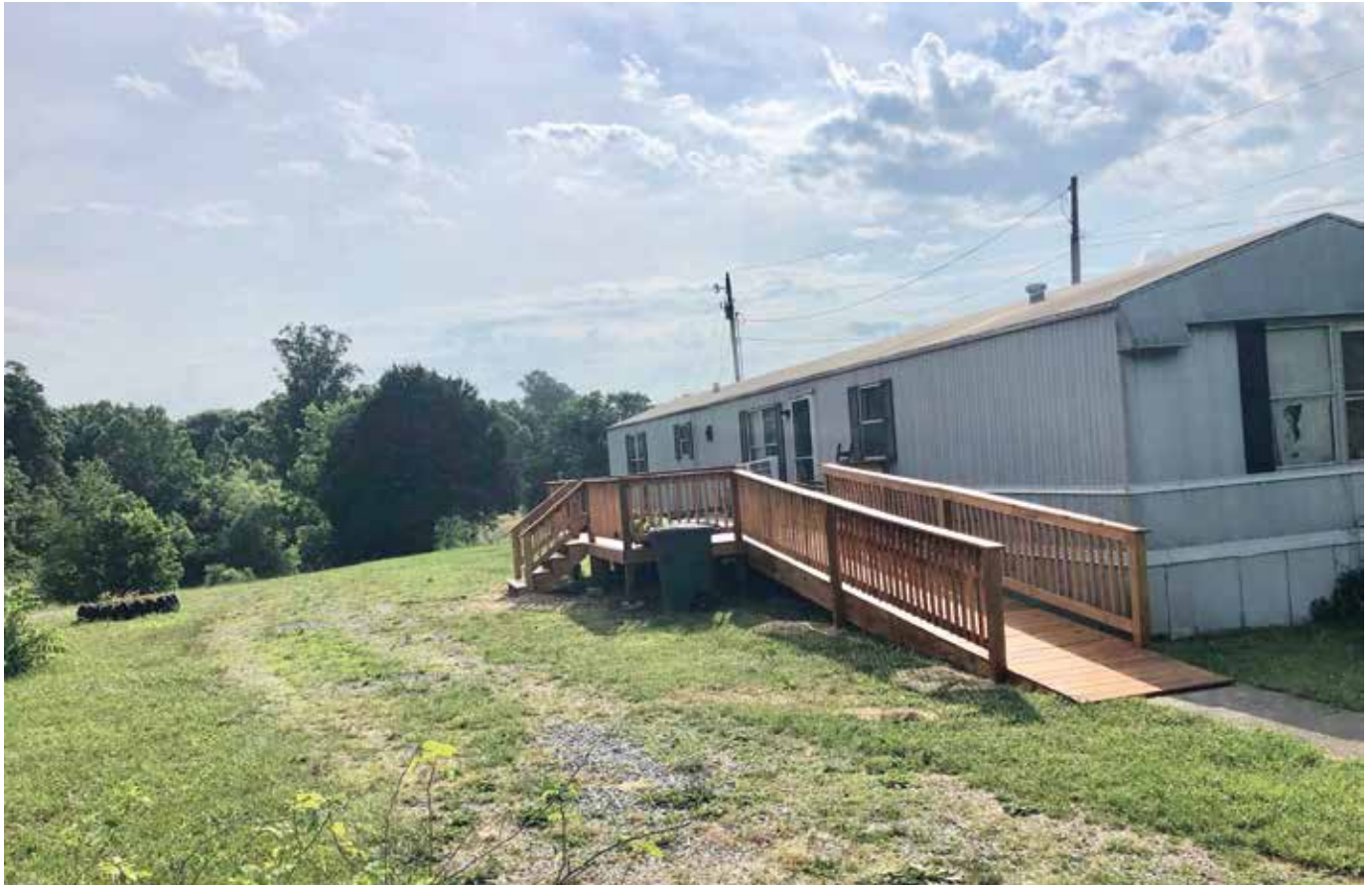
A new deck was installed for a community member during the Kentucky-Tennessee 2019 Camp Meeting.
