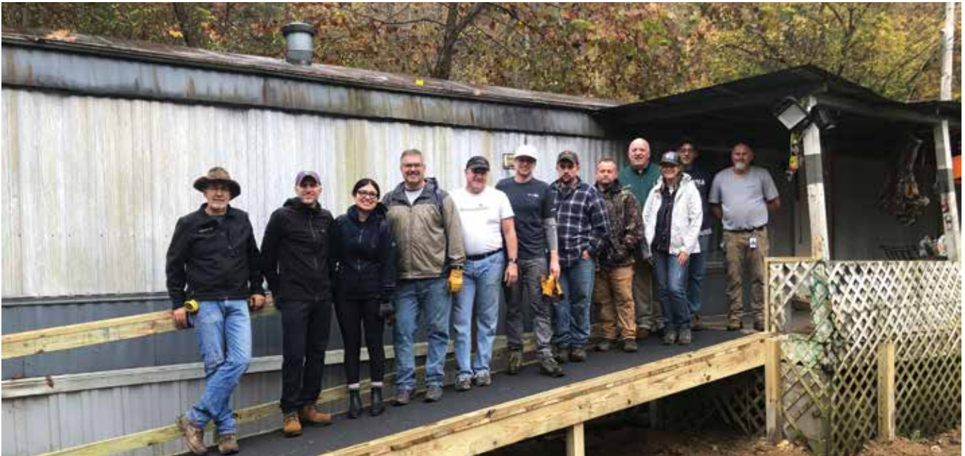
As part of the Healthy Homes project, a team from AdventHealth constructs a ramp to improve a resident’s access into their home.
