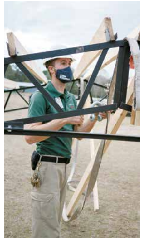
Michael Hopkins , building maintenance director at Camp Kulaqua, is shown overseeing construction of the new outdoor event pavilion.
