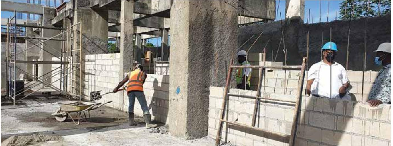
Workers at Northern Caribbean University Church lay bricks for the new building. Georgia-Cumberland Conference provided a grant to help fund this project, recognizing how important NCU is to Conference pastors and members.
