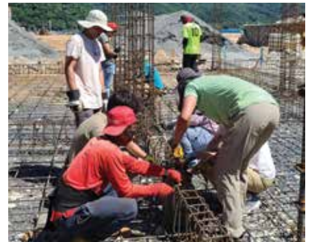
Collegedale Academy students spent their spring break helping to rebuild the Adventist school in Bonacca, Honduras. The school, along with parts of the English-speaking church, had previously burned down.
