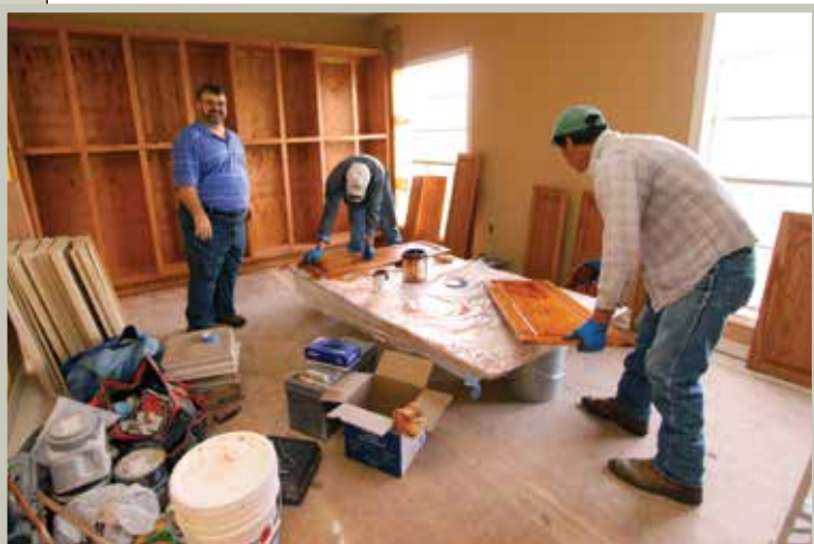
▲ Mike Agee (left), new general manager of KJRN “The Journey” 88.3, helps with the construction of the new radio station at Southwestern Adventist University.
