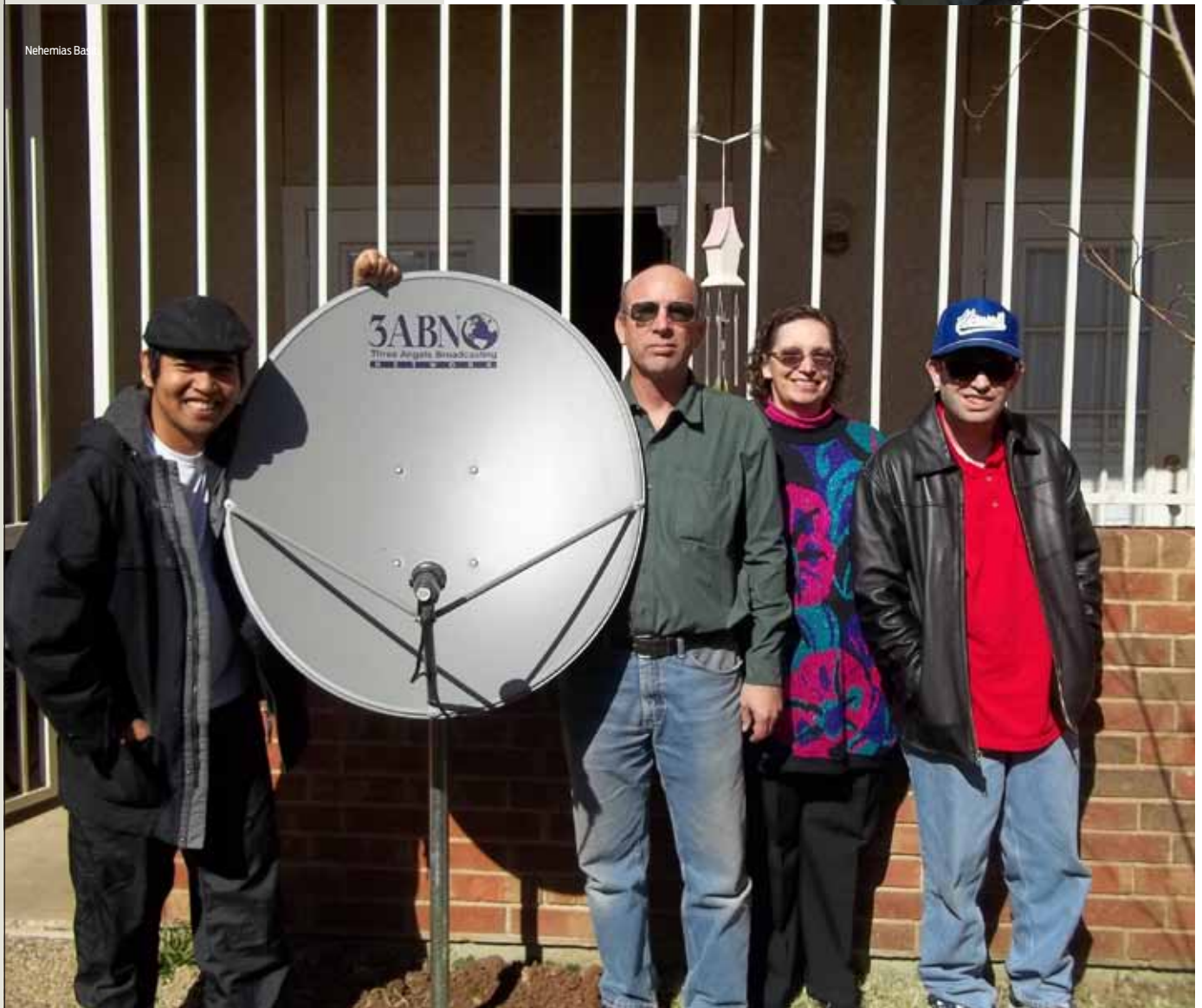
From left: Byrne Querol with Harry, Mary, and Joe Stone, as they happily show the finished satellite installation.
