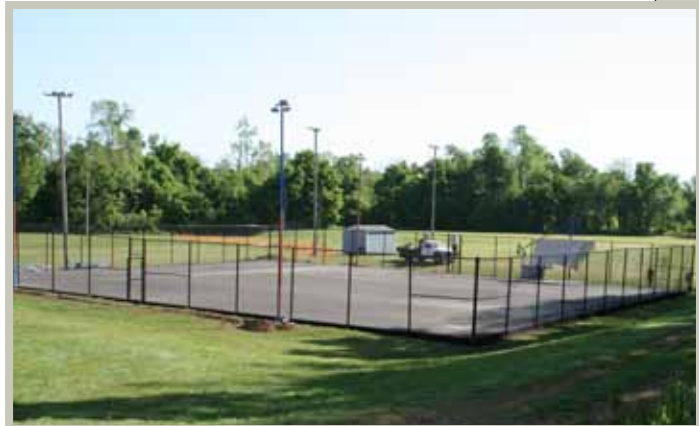
▲ The new Davis Tennis Courts in the construction process. ▼ Students during Academy Days at Ozark Adventist Academy.
