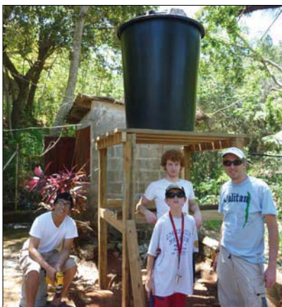
JJ Lao, Alex Roddy, Michael Davidson, and Liam Davidson construct a water tower. The rainwater collected in it will flush toilets at the Camp Bay School.
